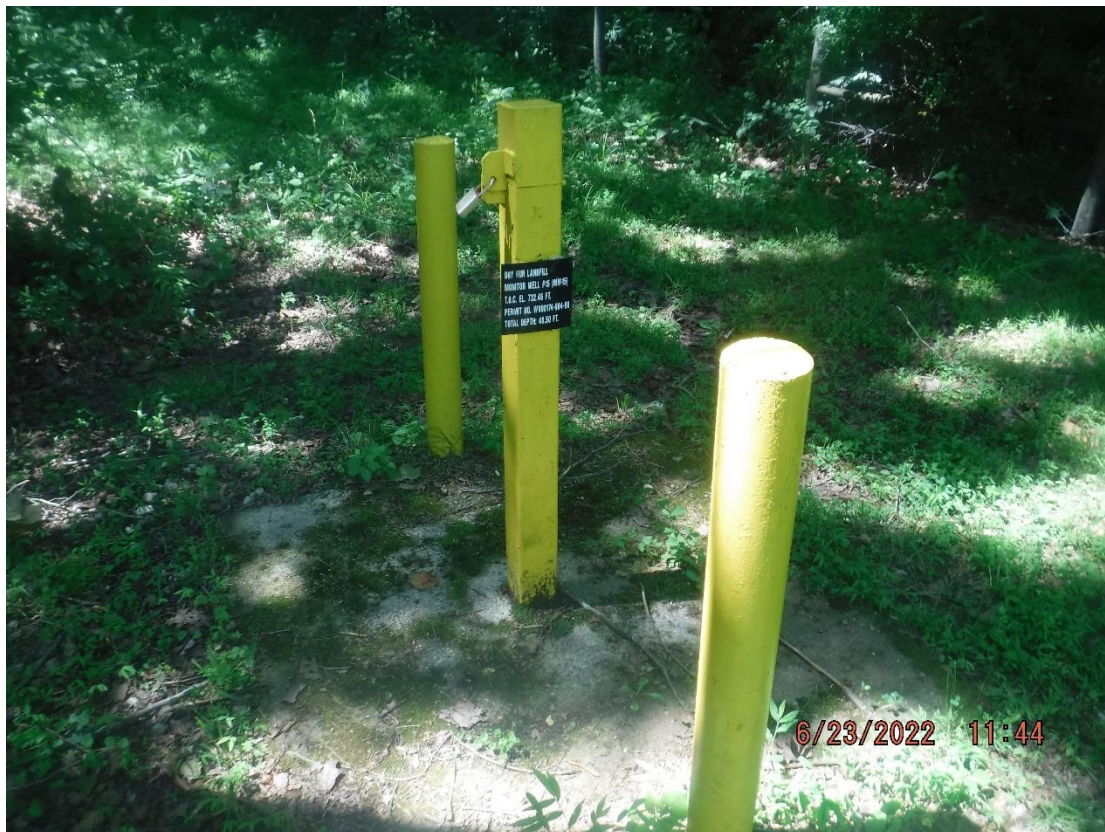
MW 15, monitoring wells observed during the inspection were found to be in good condition - 6/23/2022 11:44 am
