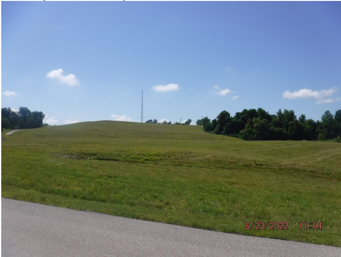
Landfill overview, no issues with final cover were noted during the inspection – 6/23/2022 11:04 am
