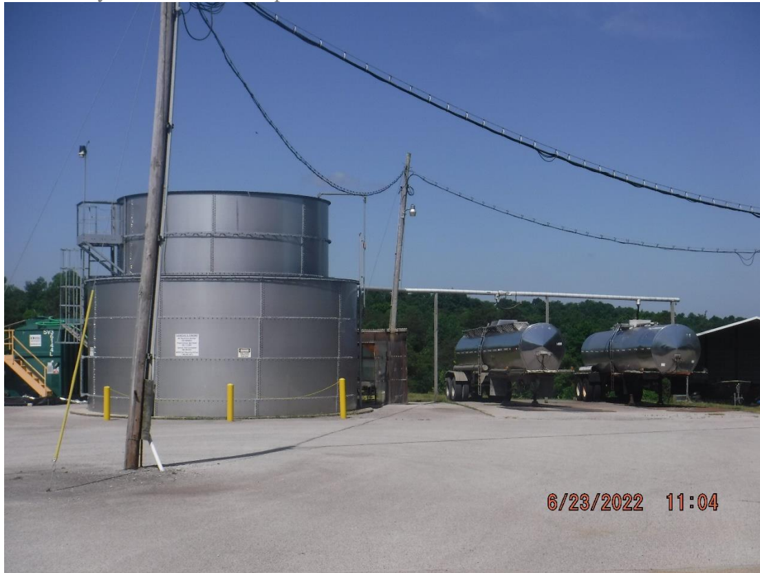
Leachate above ground storage tank was found to be leaking after seals were compromised during a cleaning. Plans are in place to replace leaking seals – 6/23/2022 11:04 am
