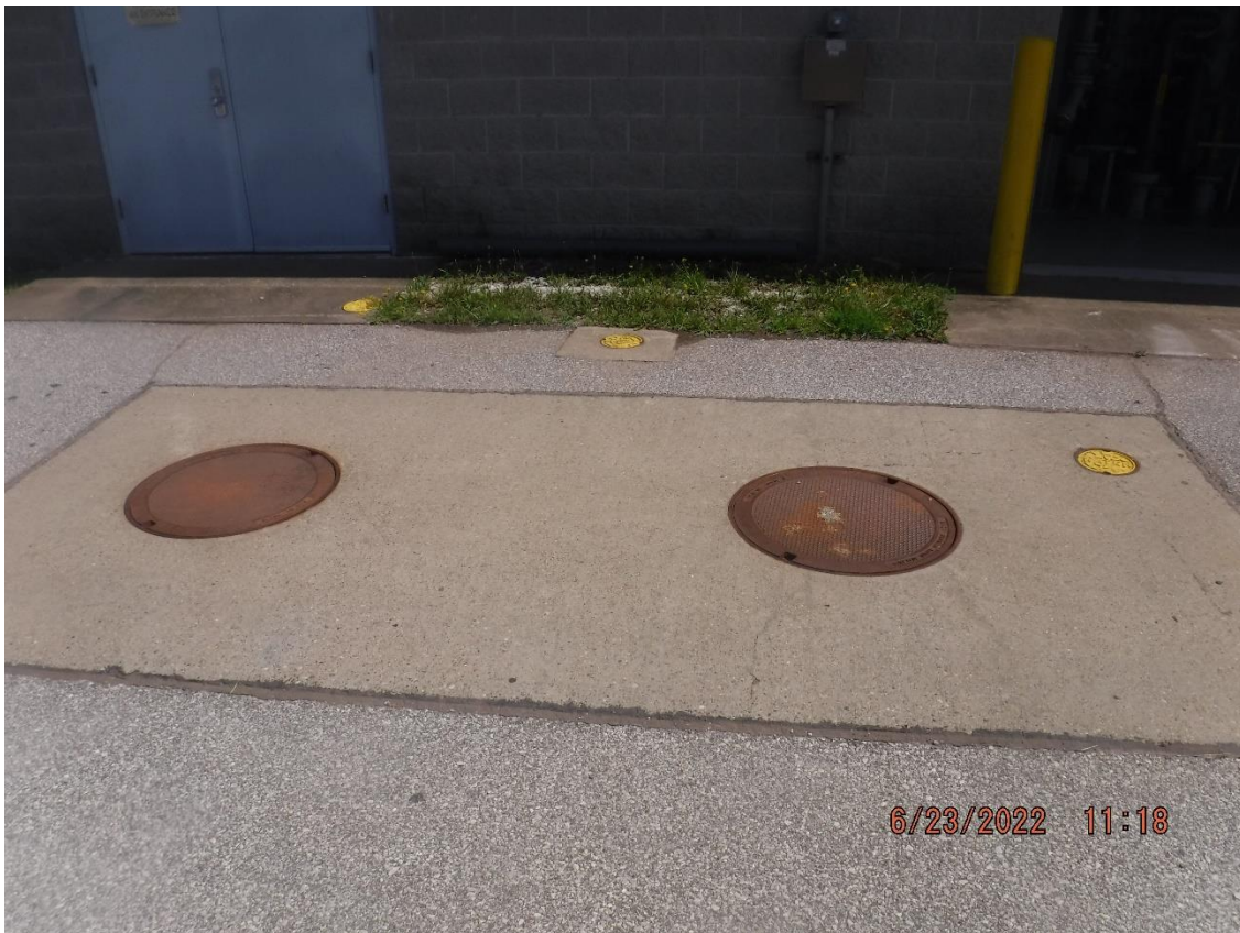
5,000 gallon underground treated leachate storage tank, tank discharges to outlet 006 – 6/23/2022 11:18 am
